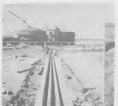
THE TWO lines run a distance of 4400 feet from the storage tanks to the blending plant. Many cubic yards of coral and earth had to be excavated so that the lines could be protected in trenches.
